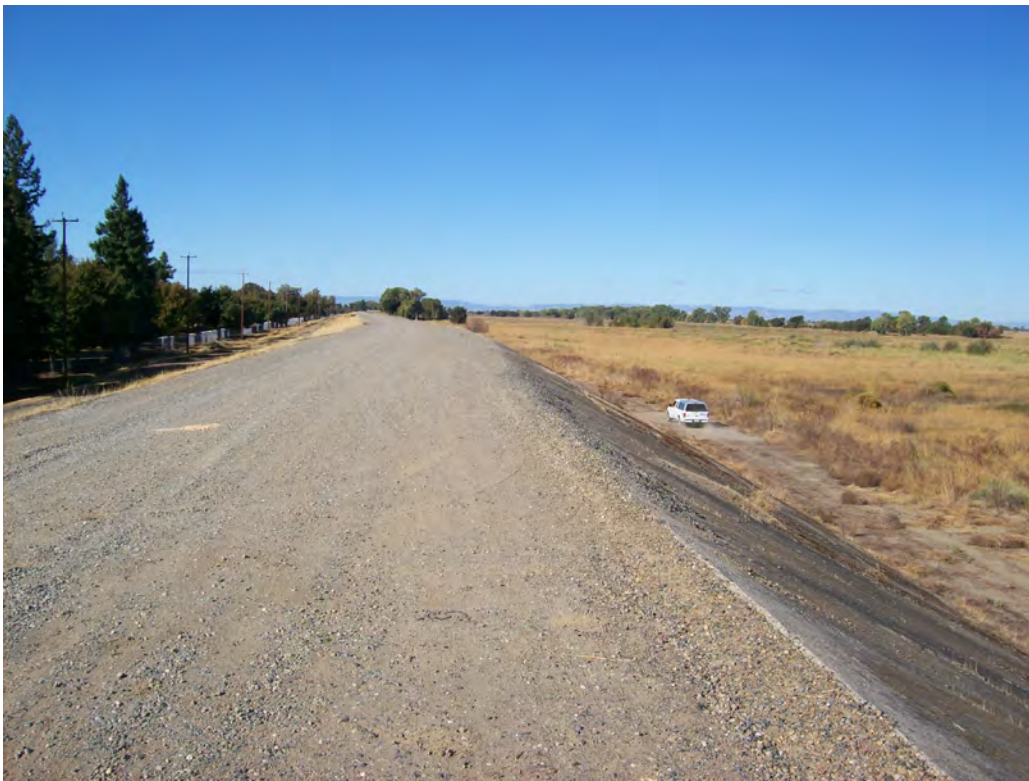
Looking west on the levee crown. Note fence, overhead utility lines, and trees at left, marking the boundary of the CHP Academy facility to the south. Sacramento Bypass is at right, north of the levee. Note concrete liner on the levee slope in right foreground.
