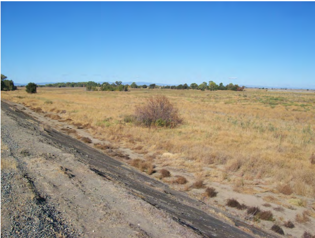
Waterside slope of Sacramento Bypass Levee looking northwest. Note mature vegetation on bypass floor along horizon.
