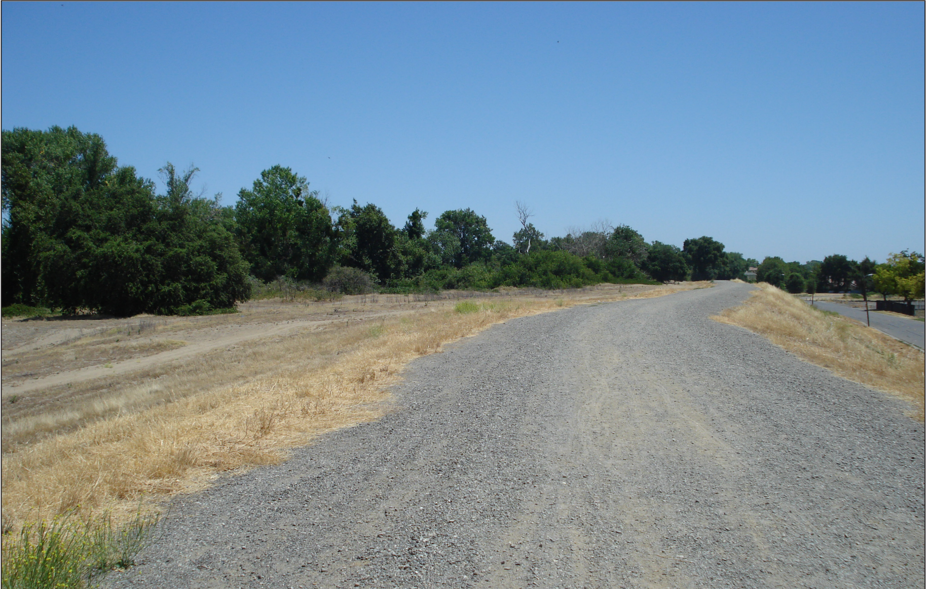
Looking due east from atop the levee crown, west of The Rivers community. Note the very wide levee crown, and the row of riparian vegetation in the middleground to the north.
